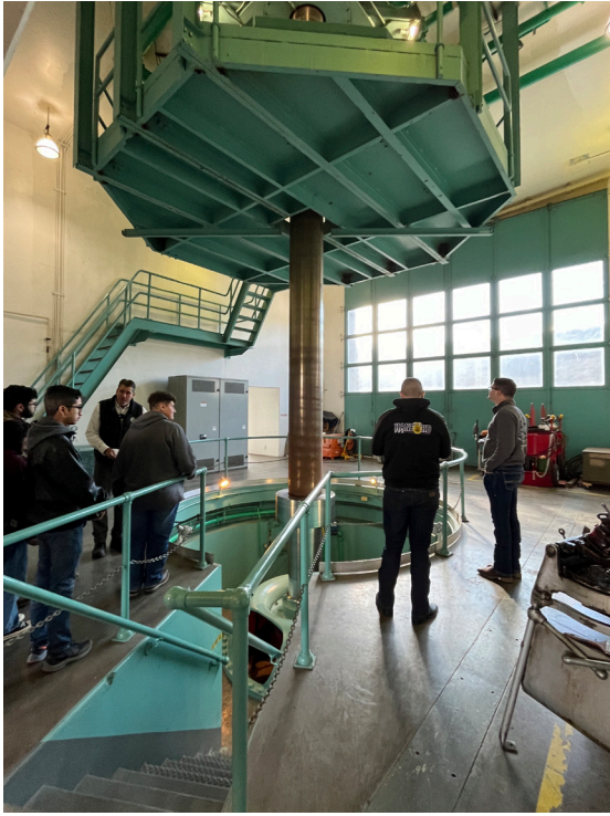
Jones Pumping Plant
