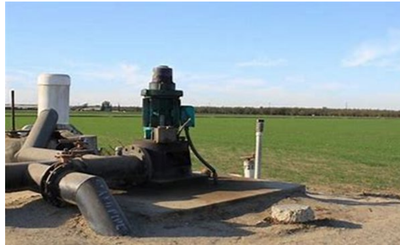
Groundwater Pumping Station
